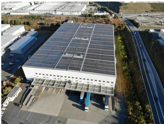
Solar panel power generation system installed on the roof of the Shinshiro-Minami Plant
