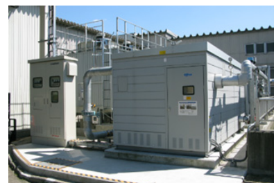
Absorption chilling equipment
