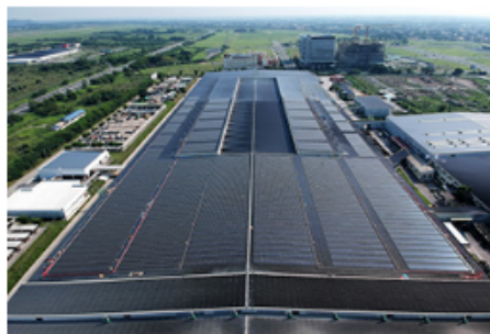
Solar power generation (Philippines) installed capacity: 4,000 kw
