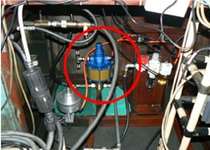
[Air hydro pumps]
