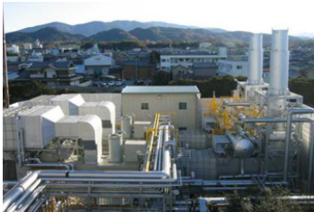
Mie Plant co-generation system
