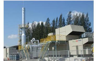
Thai Plant co-generation system
