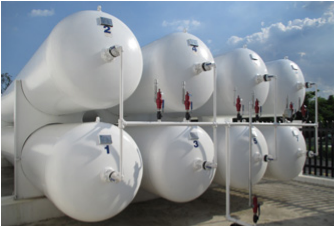
Switch to gas cylinders in the India Plant
