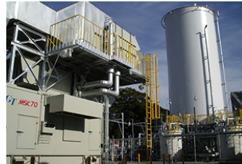
Shinshiro Plant co-generation system
