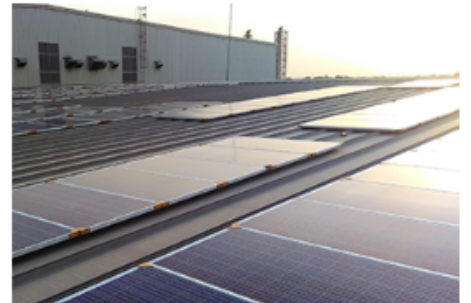
Solar power generation (India) installed capacity: 200 kw
