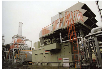
Mishima Plant co-generation system
