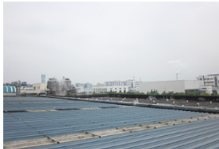
Solar power generation (Hangzhou, China) installed capacity: 80 kw
