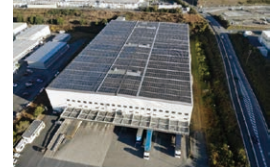
A solar power generation system installed on the roof of the Shinshiro-Minami Plant
