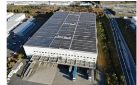
A solar power generation system installed on the roof of the Shinshiro-Minami Plant
