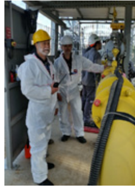
Natural gas equipment
