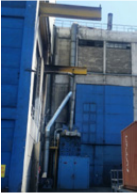
The cement house exhaust pipes (for rubber volatilization using organic solvents) have been improved.
