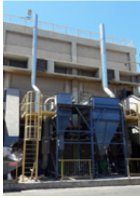
The exhaust pipes for pieces of machinery that handle chemical substances have been improved.
