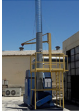
The exhaust pipe for the mixer has been improved.
