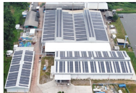
Solar panels at Thai plant
