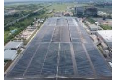
Solar power system installed at YTPi plant
