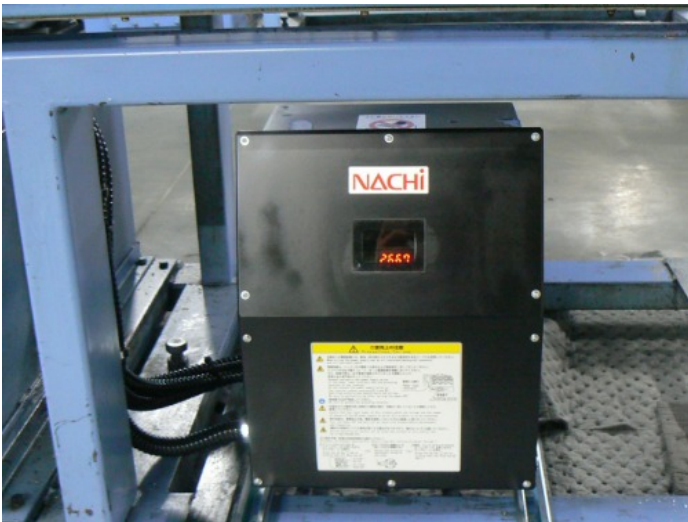
Hydraulic unit inverter conversion
