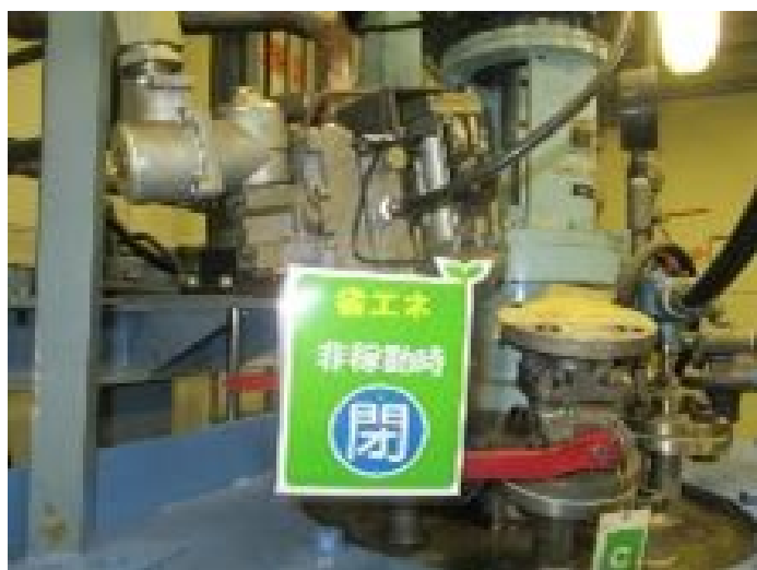
Air valve management during non-operating hours (closed)
