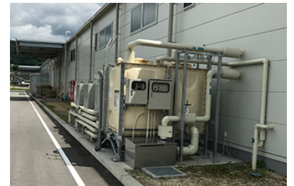
Nagano-water recycling system
