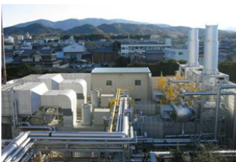
Mie Plant co-generation system
