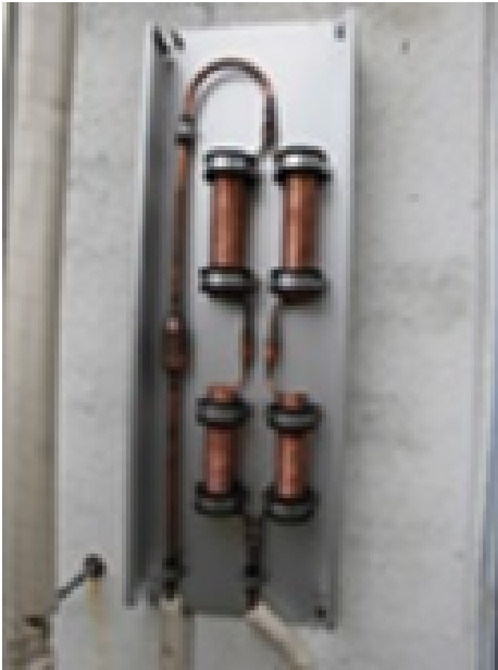
High-efficiency refrigerant liquefaction heat exchangers
