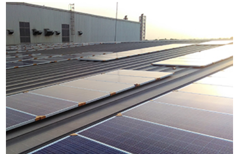
Solar power generation (India) installed capacity: 200 kw
