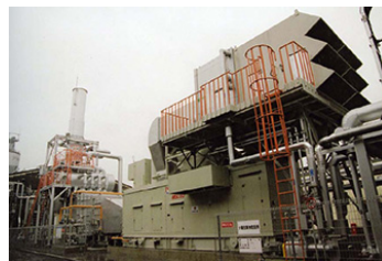
Mishima Plant co-generation system
