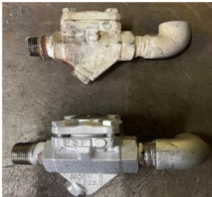
Steam drain trap (Upper photo: defective trap, lower photo: new trap)
