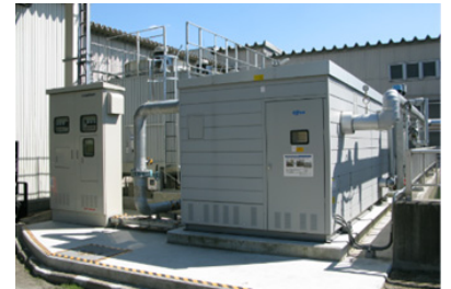
Absorption chilling equipment
