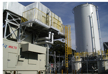
Shinshiro Plant co-generation system
