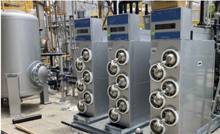
Boiler facilities Water supply system
