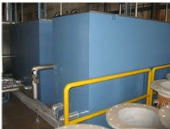
Optimizing the chiller tank
