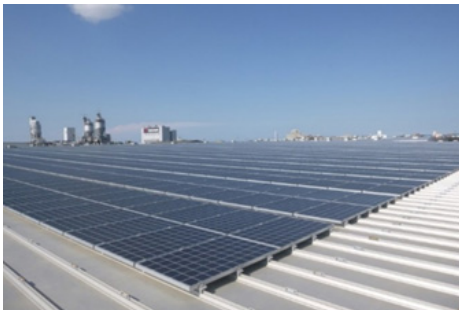
Solar power generation (Mie) installed capacity: 500 kw
