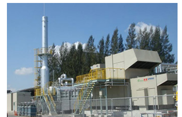
Thai Plant co-generation system
