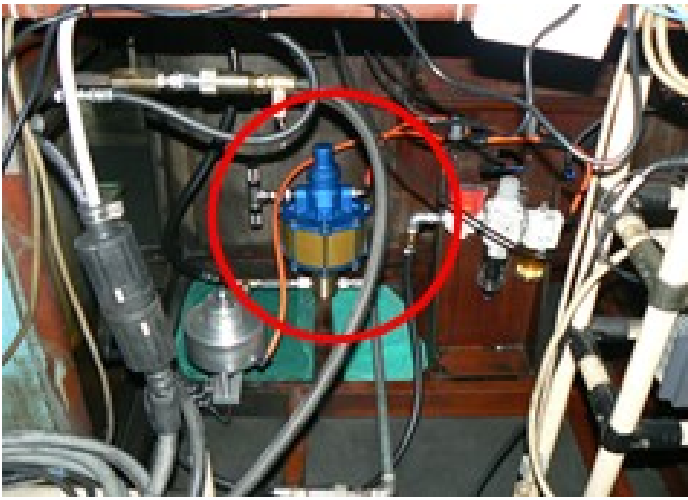
Air hydro pumps
