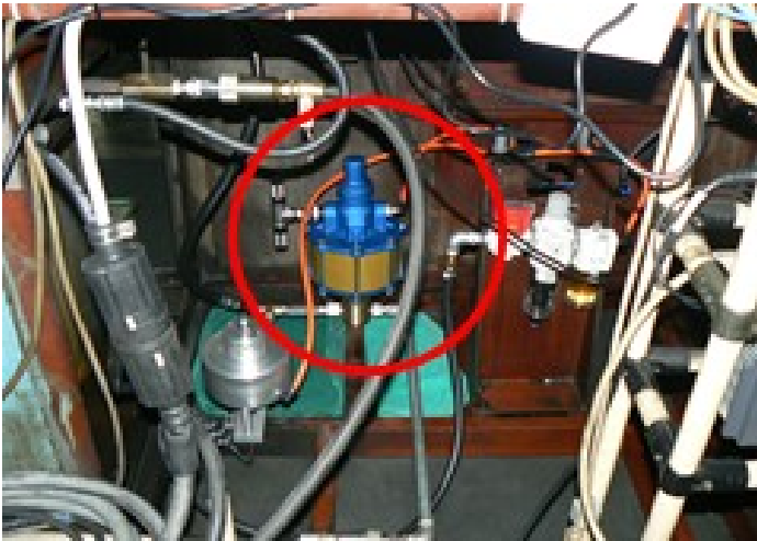
Air hydro pumps
