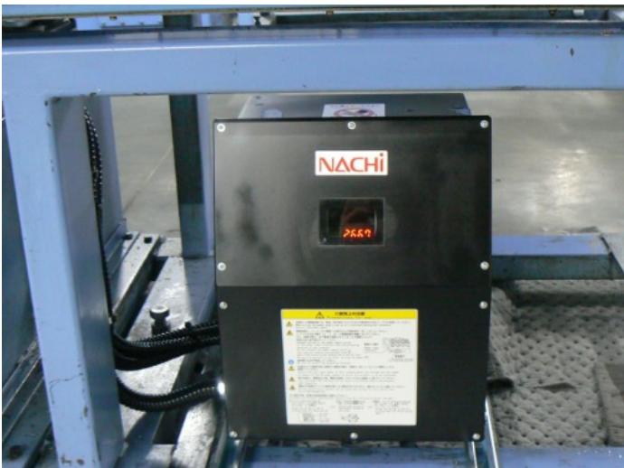
Hydraulic unit inverter conversion
