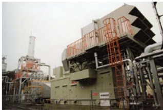
Mishima Plant co-generation system
