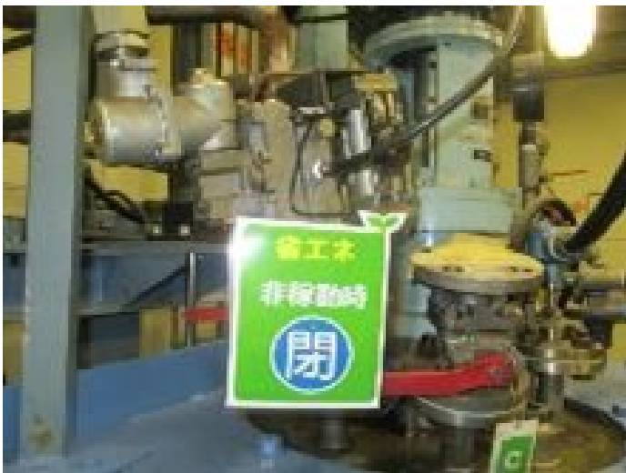
Air valve management during non-operating hours (closed)
