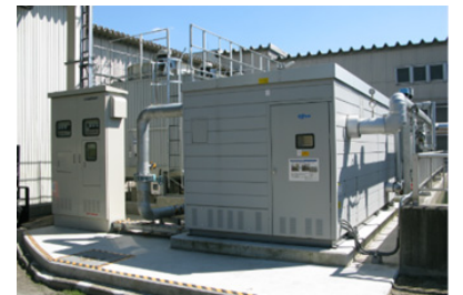
Absorption chilling equipment
