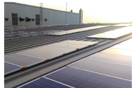
Solar power generation (India) installed capacity: 200 kw
