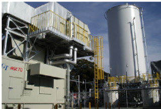
Shinshiro Plant co-generation system
