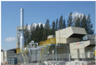
Thai Plant co-generation system
