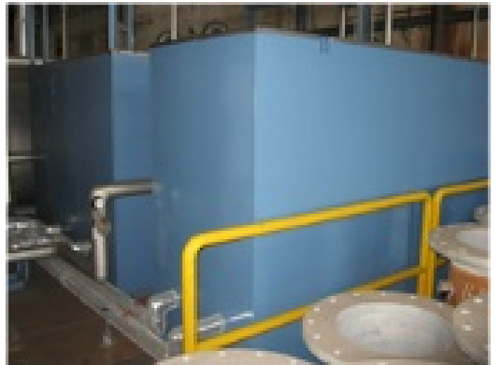
Optimizing the chiller tank
