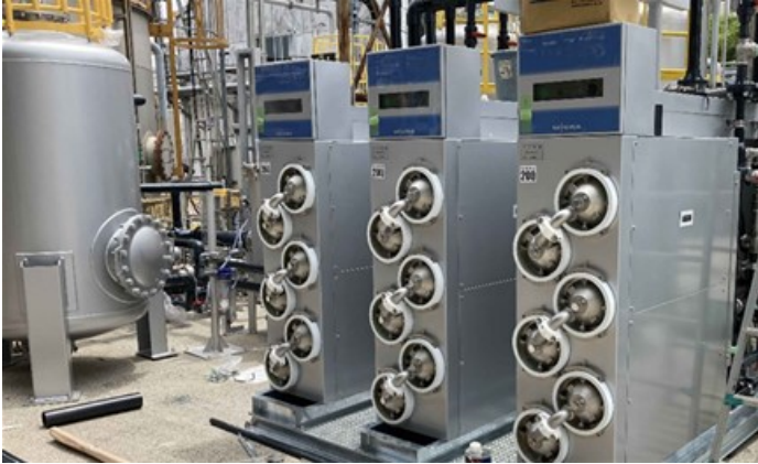
Boiler facilities Water supply system
