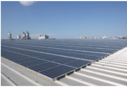
Solar power generation (Mie) installed capacity: 500 kw
