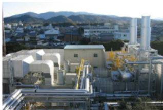
Mie Plant co-generation system
