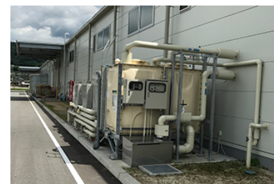
Nagano-water recycling system
