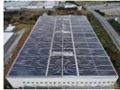
Shinshiro-Minami Plant's solar power generation facility
